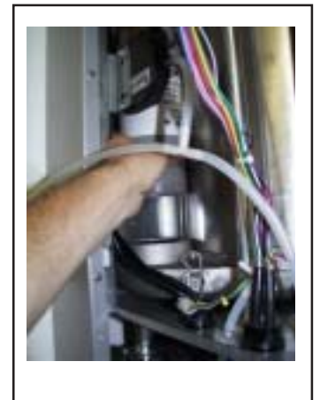
Flue pipe damper
